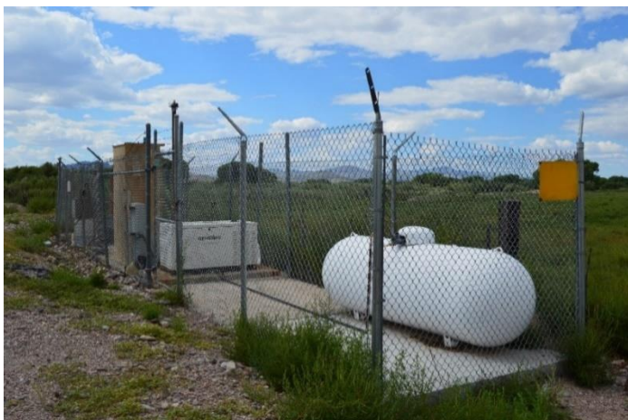
Figure 2.7-Pumping Station for Siphon
